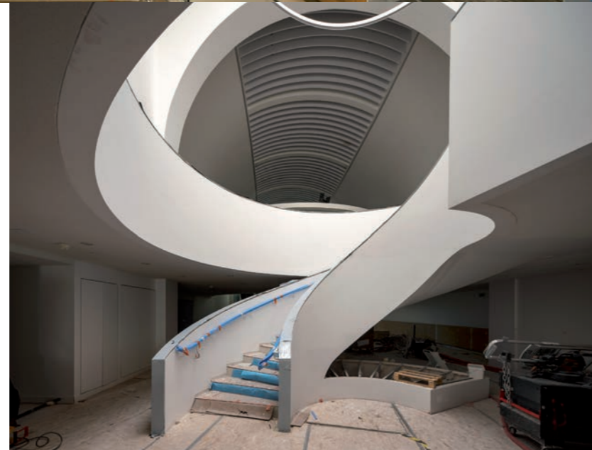
Musée National de la Marine, Paris. Renovation worksite. Palais de Chaillot. Staircase to the mezzanine in the Davioud Gallery. 04/04/2023; h2o architectes and Snehetta © Patrick Tourneboeuf/OPPIC/Tendance Floue 46
