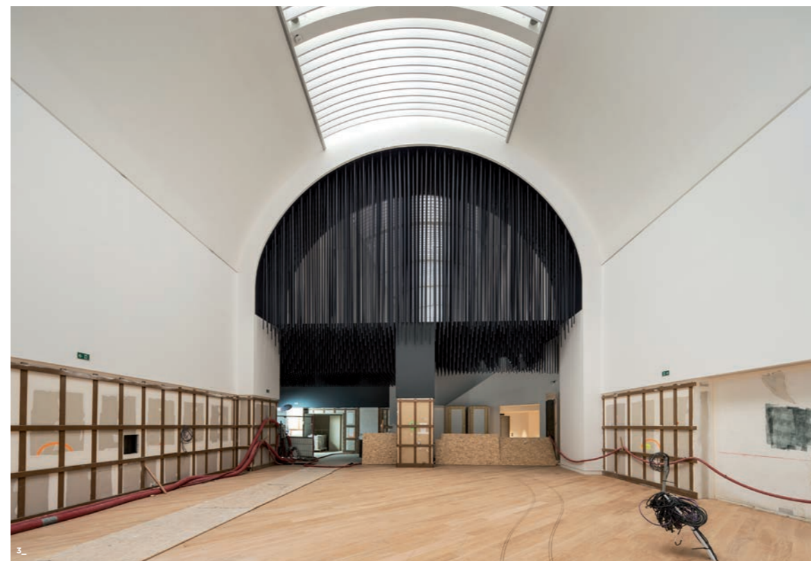
Musée National de la Marine, Paris. Renovation worksite. Palais de Chaillot; Davioud Gallery, h2o architectes and Snøhetta ©Patrick Tourneboeuf/OPPIC/Tendance Floue
