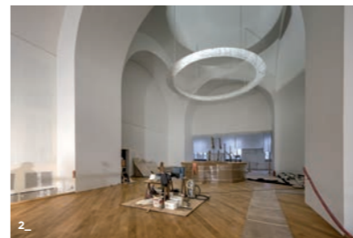
1. Musée National de la Marine, Paris. Renovation worksite. Palais de Chaillot. Davioud Gallery. 11/01/2023; h2o architectes and Snøhetta. © Patrick Tourneboeuf/OPPIC/Tendance Floue 2. Musée National de la Marine, Paris. Renovation worksite. Palais de Chaillot. Main Pavilion; Davioud Gallery. 11/01/2023; h2o architectes and Snøhetta. © Patrick Tourneboeuf/OPPIC/Tendance Floue.
