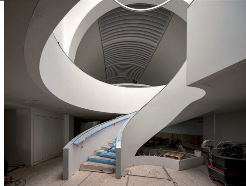
Musée National de la Marine, Paris. Renovation worksite. Palais de Chaillot. Staircase to the mezzanine in the Davioud Gallery. 04/04/2023; h2o architectes and Snehetta © Patrick Tourneboeuf/OPPIC/Tendance Floue 46
